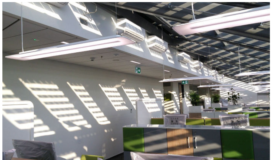
LG Wall mounted air conditioners units: indoor offices.
